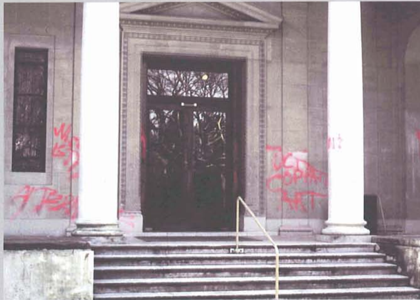
Graffiti damage to the Gallery in the early 80's.
