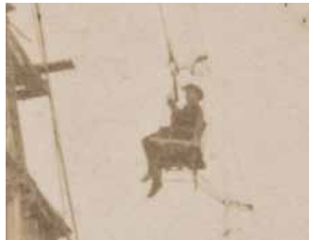
Above and detail: Edward Wheeler Bishop Julius being hoisted to lay the coping stone on Christ Church Cathedral spire, 5 August 1891. Albumen photograph. Smith's Bookshop Archive
