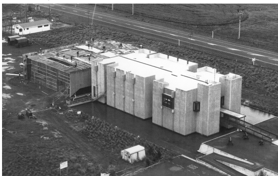
STAGE 2 UNDER CONSTRUCTION, THE FIRST ADDITION TO THE ORIGINAL BUILDING. ACKNOWLEDGEMENT: QUEEN ELIZABETH II ARMY MEMORIAL MUSEUM
