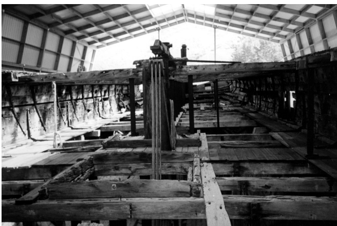
RAINWATER RAVAGED DECK BEAMS EXPOSED AFTER THE TEAK DECKS WERE STRIPPED DURING THE SHIP'S 19-YEAR BEACHING IN SHAKESPEARE BAY HAVE BEEN SPECIALLY TREATED TO PREVENT FURTHER DETERIORATION. ACKNOWLEDGEMENT: THE EDWIN FOX SOCIETY
