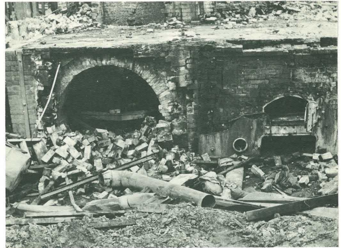
Sawmill Dutch oven boiler fireboxes in stages of demolition after 35 years of use. Note the forced draught duct and the wood-ash-glazed bricks at the back of the uptake throat photo: Ron Cooke
