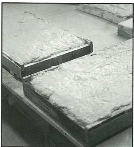
7: As the water is absorbed the mix will shrink and compress from three-eighths to one quarter of an inch thick
