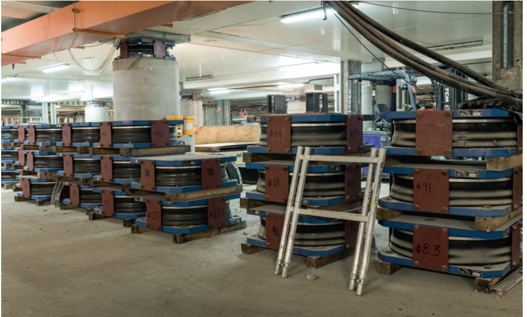
Base isolators stacked in the basement
