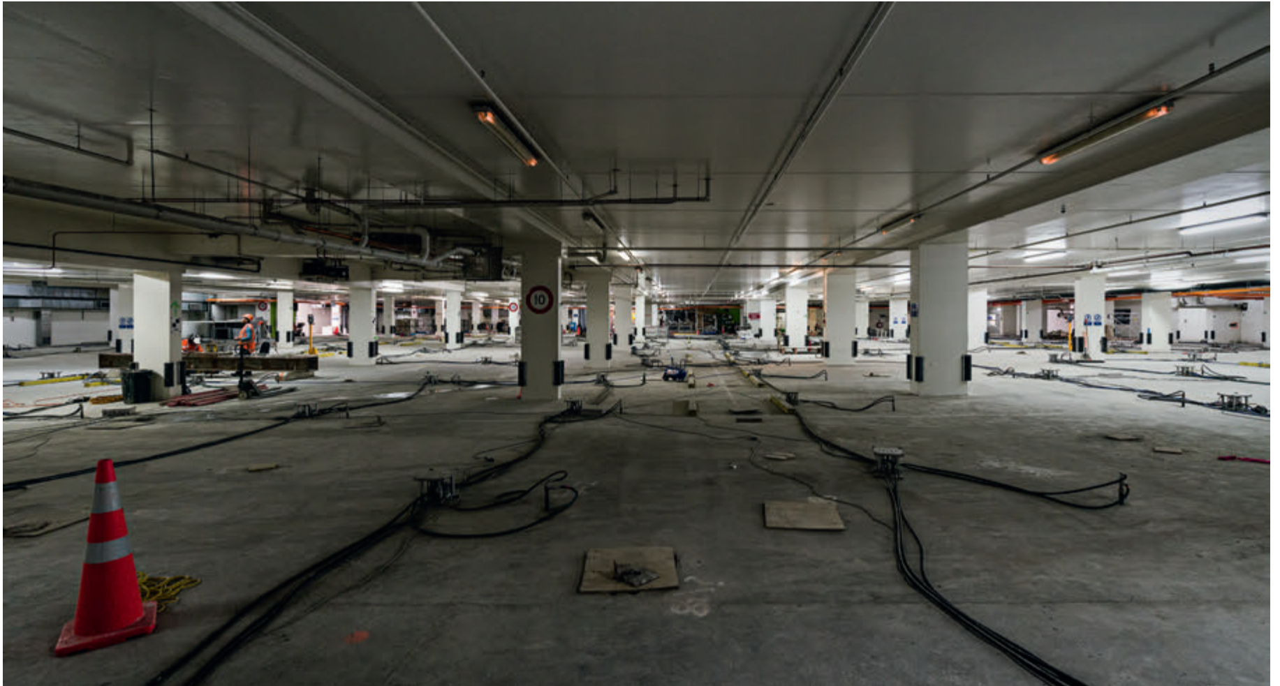
The robotic stations monitoring the movement of the building during the re-levelling process
